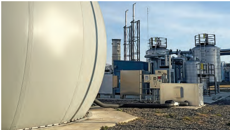
The Gloucester County Utilities Authority's biosolids process transformation includes the first egg-shaped digesters in New Jersey. The egg shape eliminates dead corners where undigested biosolids can accumulate.
